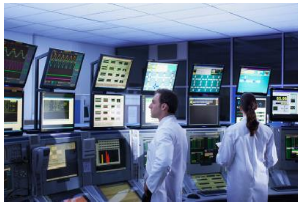
Hub Commination's Room
